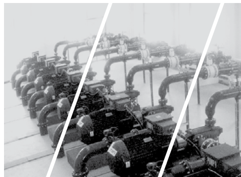
Boosting and Distribution of surface water
