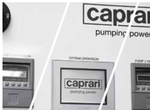
Pump Control Technology
